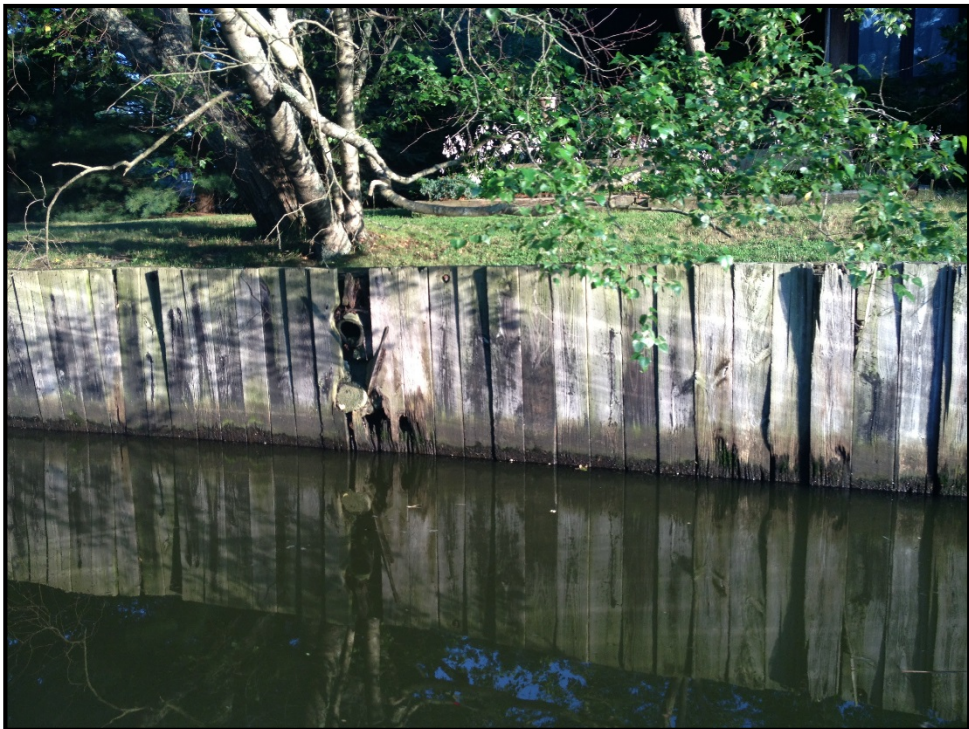
Portions of bulkheads along the canal shoreline on private property are in severe disrepair.
