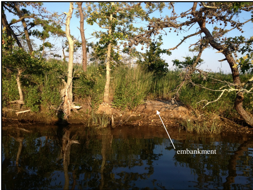
The embankment which separates the canal from the wetland areas is restricted with trees, many of which have exposed roots from erosion.
