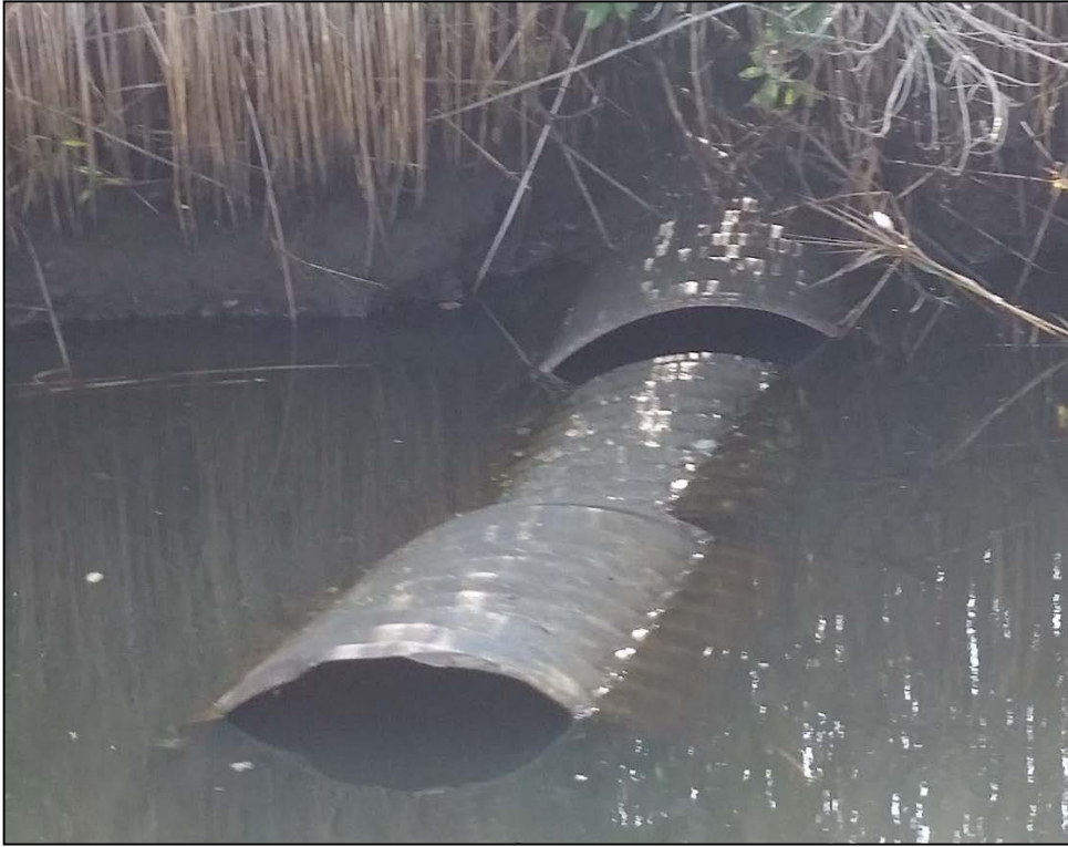
Culverts in poor condition provide little tidal exchange between canal and bermed wetlands.
